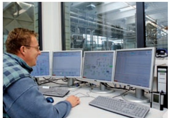
Process control room of a multi-effect fully automated evaporation plant
