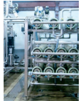
Membrane filtration plant
