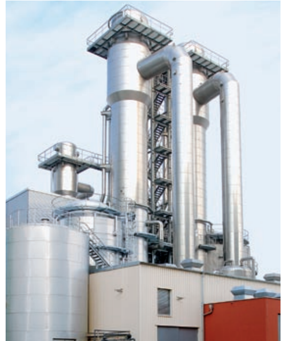
Concentration of potato juice Two pre-evaporators with mechanical vapour recompression and a finisher with thermal vapour recompression. Evaporation rate in total: 152,000 kg/h
