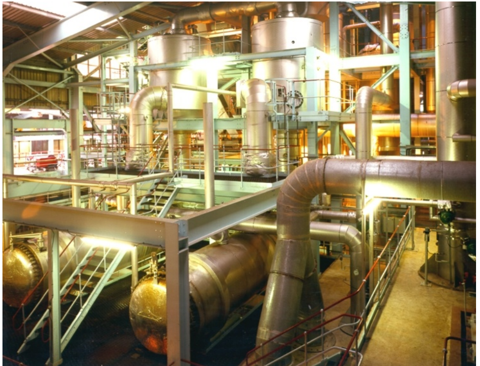
Fig. 5: 4-effect falling film and forced circulation evaporator, heated by mechanical vapour recom- pressor, concentrating 125 ton- nes/hr of whisky stillage, as per arrangement B (flow sheet in fig. 6)
