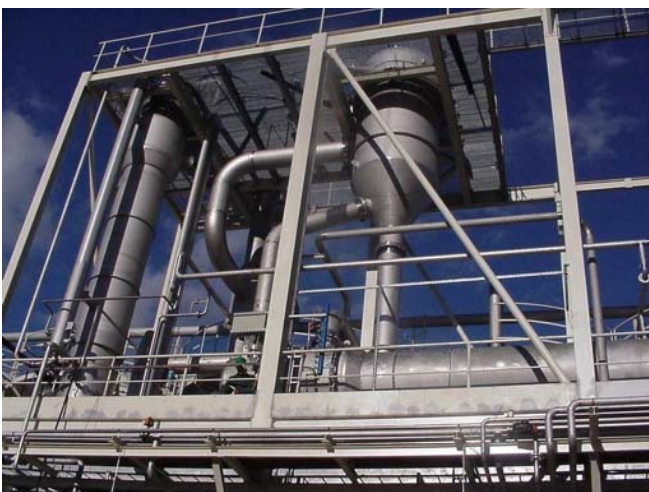
Fig. 4: 5-effect falling film and forced circulation evaporator, heated by thermal vapour recompressor, concentrating 30 tonnes/hr vinasses, arrangement A
