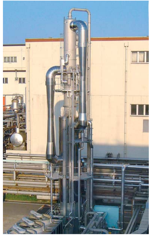
Fig. 7: 2-stage steam jet cooling plant of column design, cooling 200 m 3 /hr of water from 10 to 5 °C. Chilling capacity: 1163 kW
