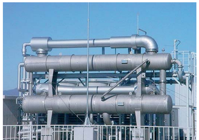
Fig. 5: 2-stage steam jet cooling plant of compact design, cooling 44 m 3 /hr of water from 30 to 10 °C.
