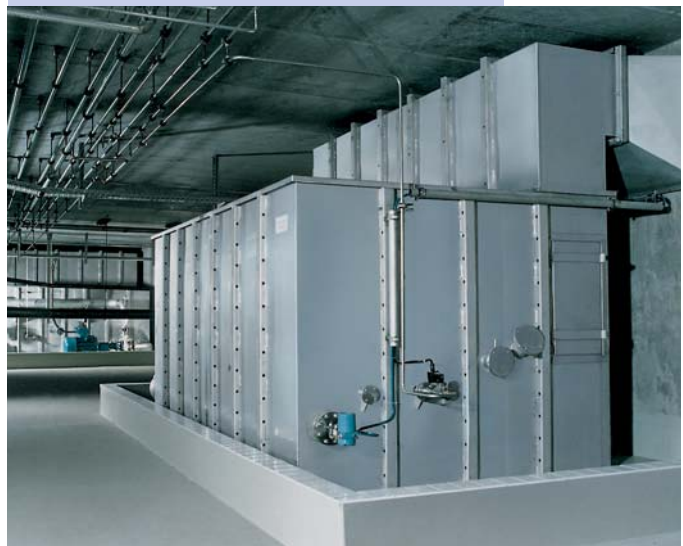
Jet scrubbers for the separation of colour mist from a paint shop for commercial airplanes.
